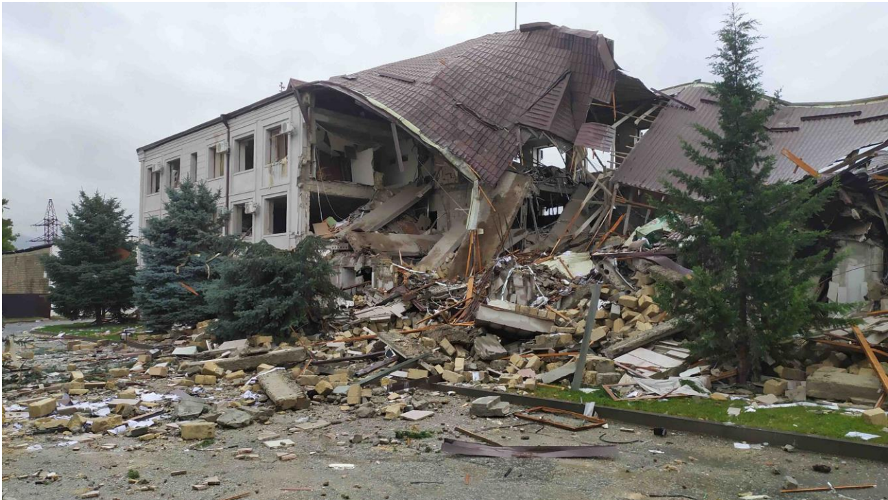
Figure 16. The Head Office of “Artsakh Energy” Company after Being Struck by Azerbaijan
