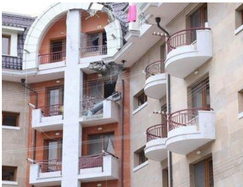
Figure 32. A Part of Azerbaijani Missile on a Residential building of Stepanakert City
