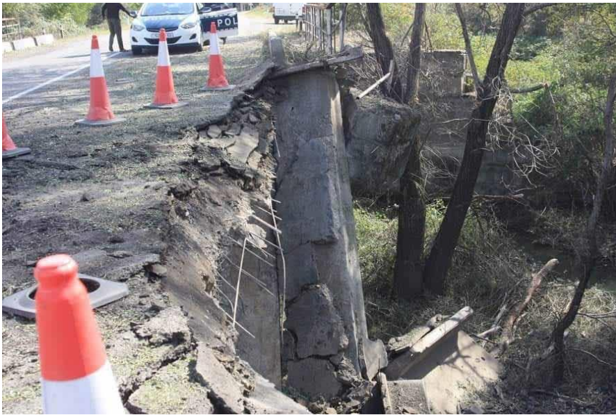
Figure 21. A Bridge in Berdzor after Being Struck by Azerbaijan
