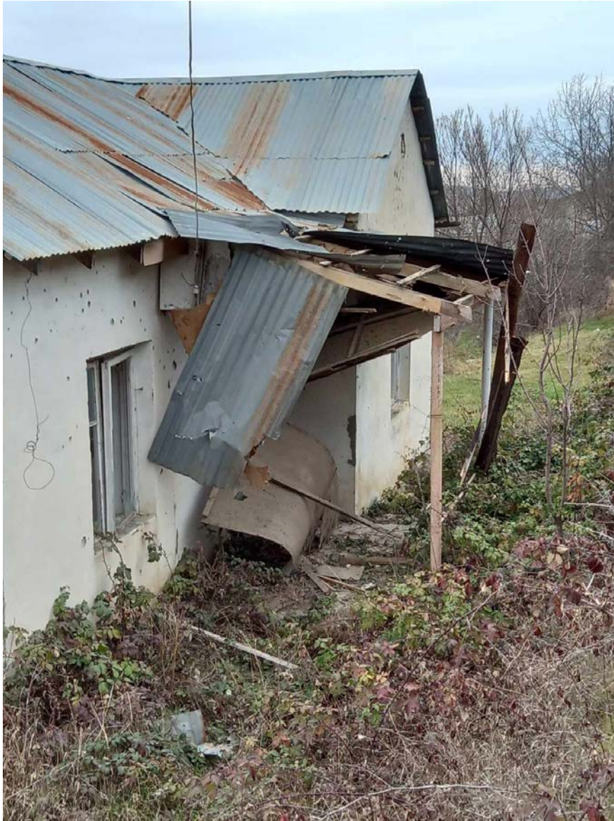
Image 2 . Damaged community building in Parukh village
